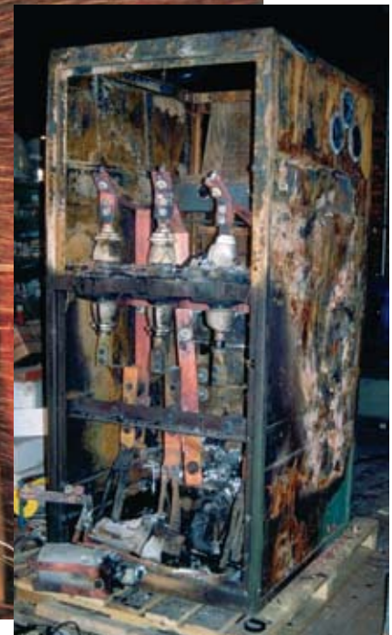
Damage caused to medium voltage switchgear by an arc fault
