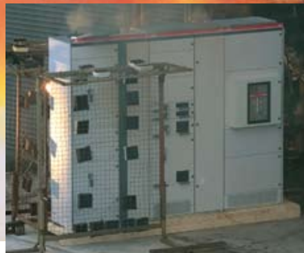
Low voltage switchgear during test
