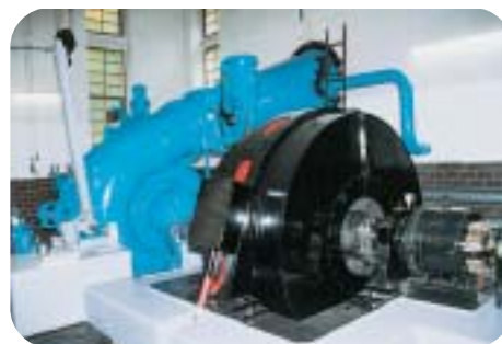
At pumping stations
