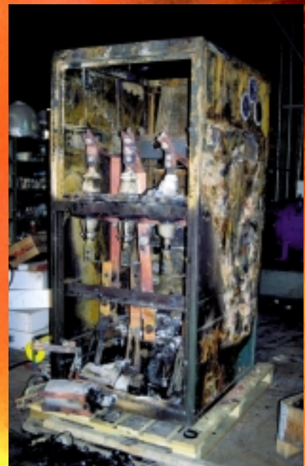
Damage caused to medium voltage switchgear by an arc fault (SE902001)
