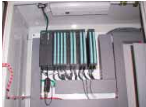
"After" — Adopting modular solutions for control panels requiring more than 200 I/O points gave the systems a more aesthetic appearance, provided a faster, more reliable assembly, and eliminated most wiring labor costs.
