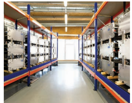
The redox-flow large-battery storage facility at the Fraunhofer ICT in Pfinztal: the pilot system is equipped with Schmalz stacks.
